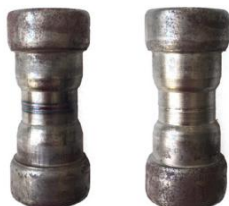
Water Pipe Joint
